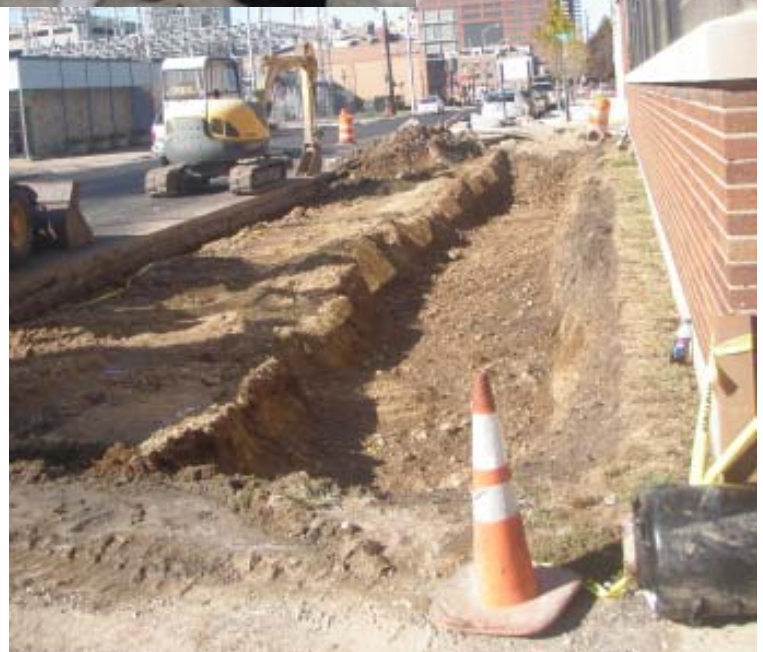
IN PROCESS: Rain garden taking shape. Plant material will be planted in spring 2011.
